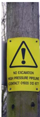
Pole warning marker
